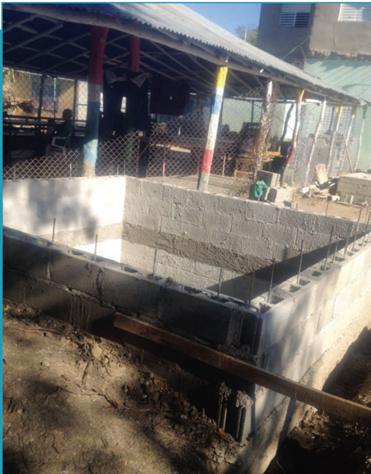
Left: The progress in the construction following the sketches or design originally submitted can be seen here as walls are laid atop the foundation.
