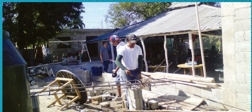
Right: A construction worker manipulates rebar that will be used to strengthen the load-bearing walls of the new structure.
