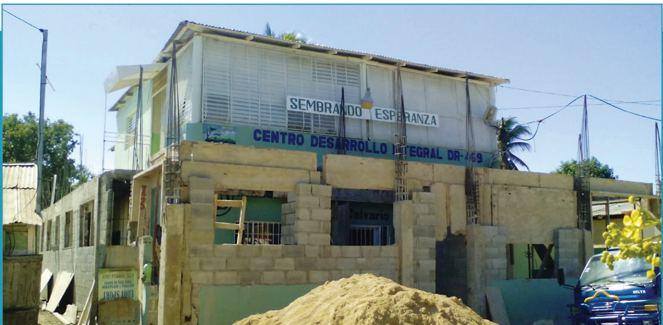
Above: The original front façade of the center can be seen here behind the new construction.
